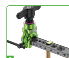
2 The copper pipe enters the hole, and the limit plate is on the copper pipe
