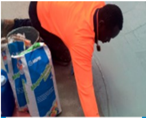
Installing Mapelastic Smart in the 50 metre pool at the Adelaide Aquatic Centre
