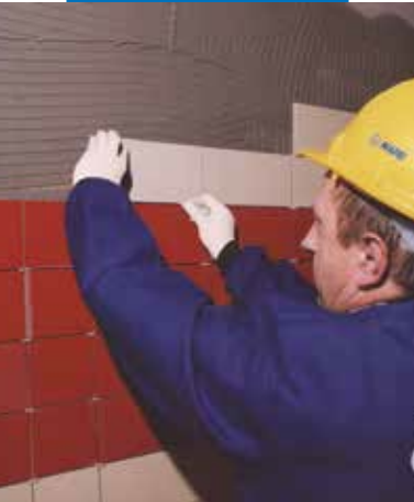
Fixing ceramic tiles on walls working from the top to the bottom
